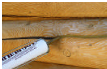
Fill checks and cracks.
